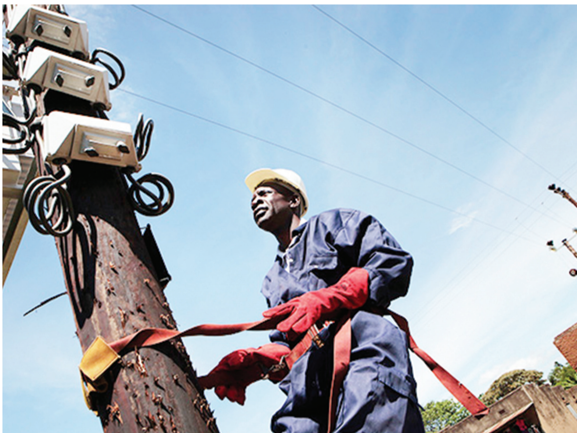
An electrician at work. The public will spend slightly less on power after ERA reduced tariffs
